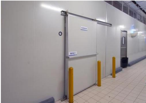
Cold room 冷库
